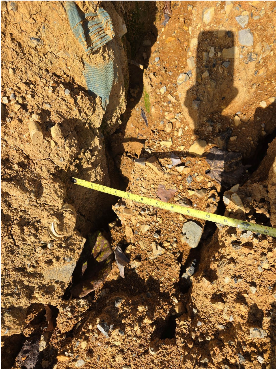
Figure 15 – Settlement Crack within the Quarry
