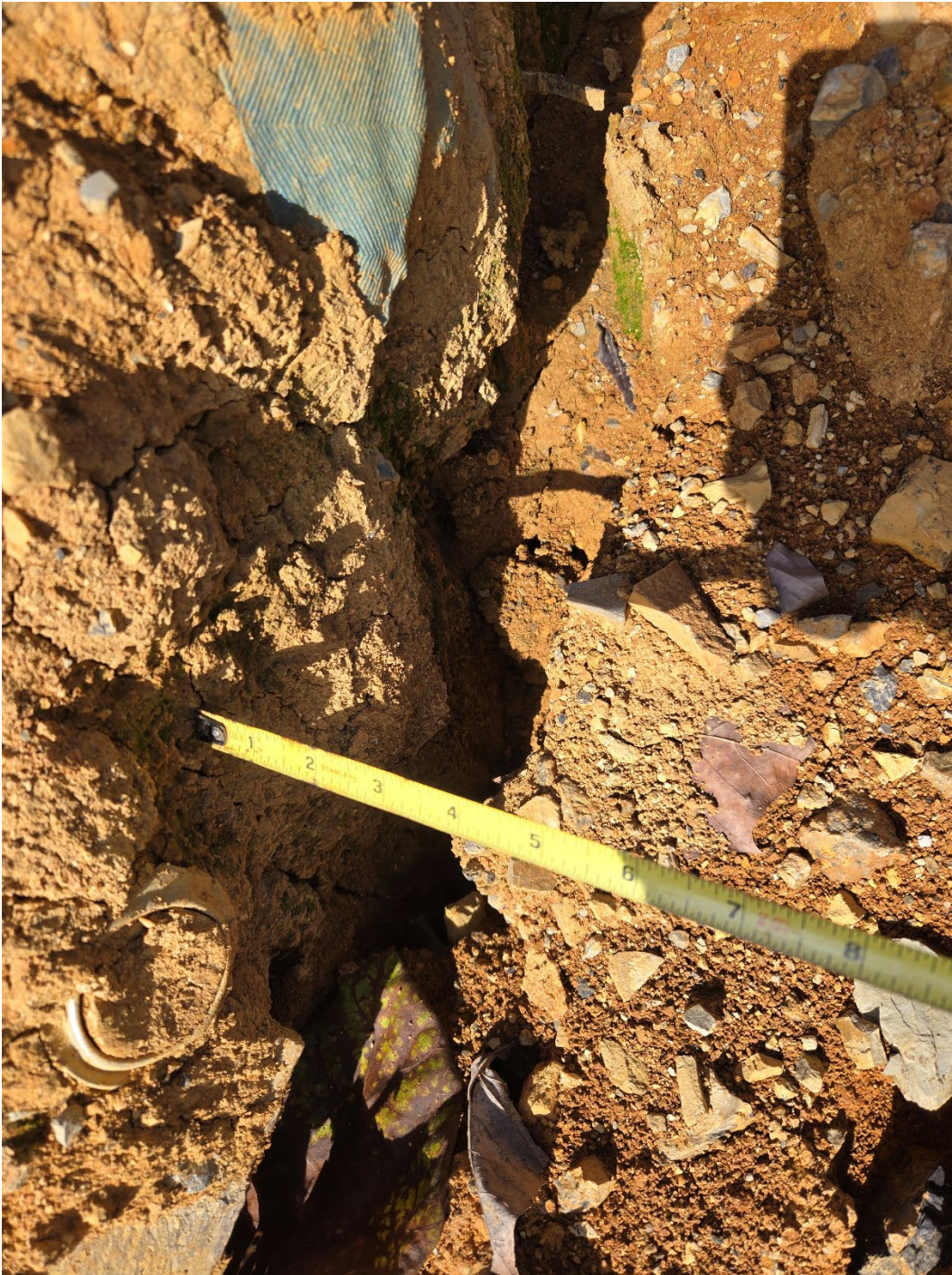
Figure 16 – Settlement Crack within the Quarry
