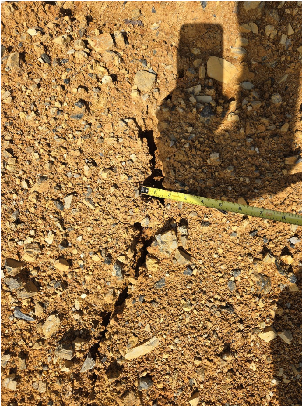
Figure 14 – Settlement Crack within the Quarry
