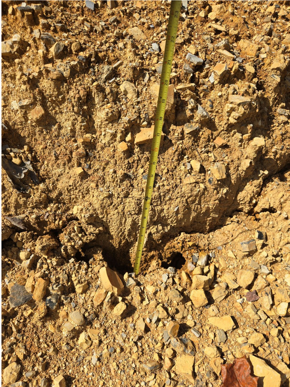
Figure 17 – Settlement Crack within the Quarry
