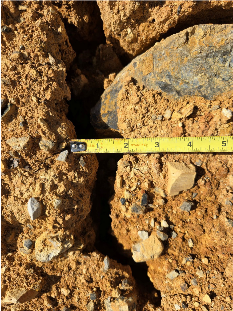
Figure 18 – Settlement Crack within the Quarry
