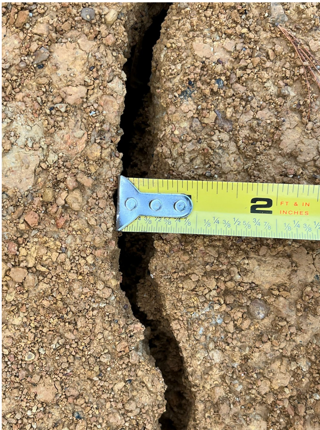
Figure 15 – Settlement Crack Observed in Southwest Area Near Sidewall Bench
