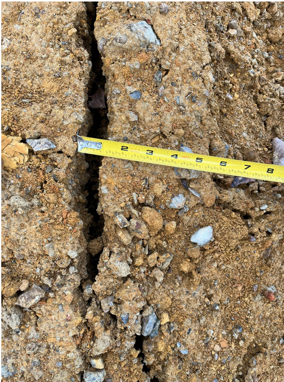
Figure 14 – Settlement Crack Observed in Southwest Area Near Sidewall Bench
