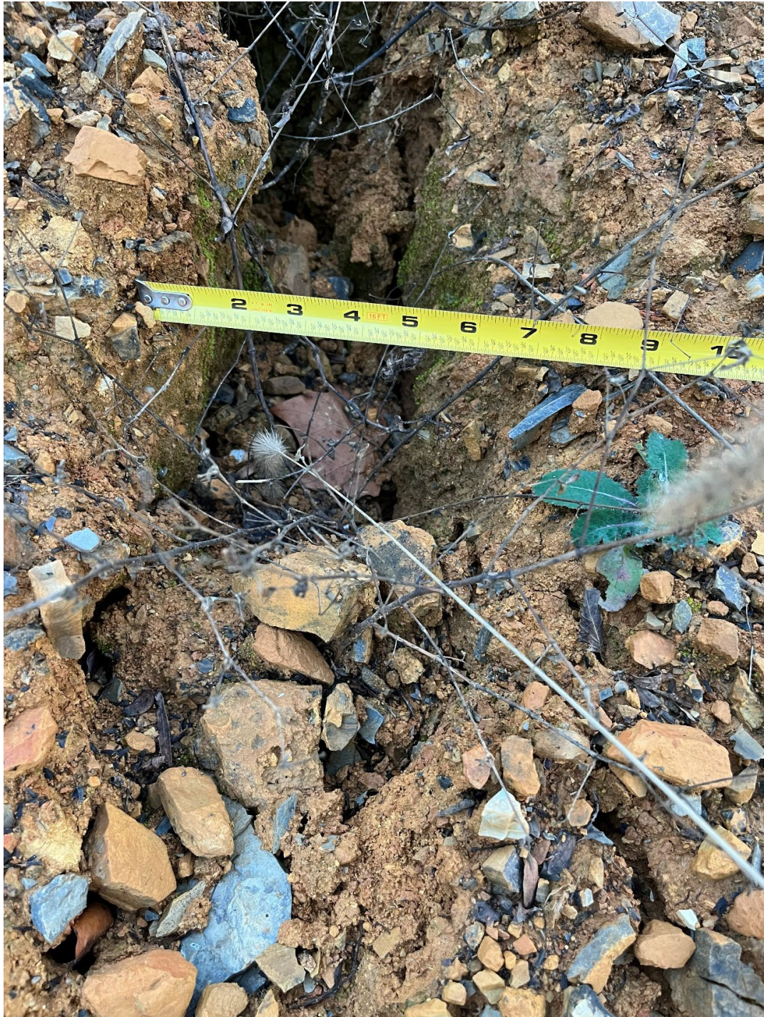
Figure 18 – Settlement Crack Observed in Northern Area Near the Access Road Entrance
