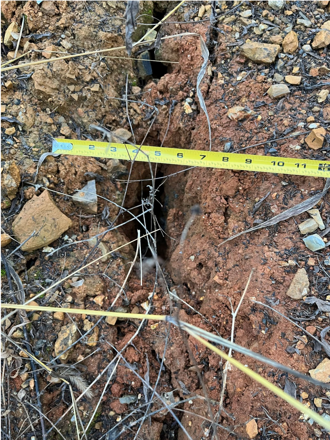
Figure 17 – Settlement Crack Observed in Northern Area Near the Access Road Entrance
