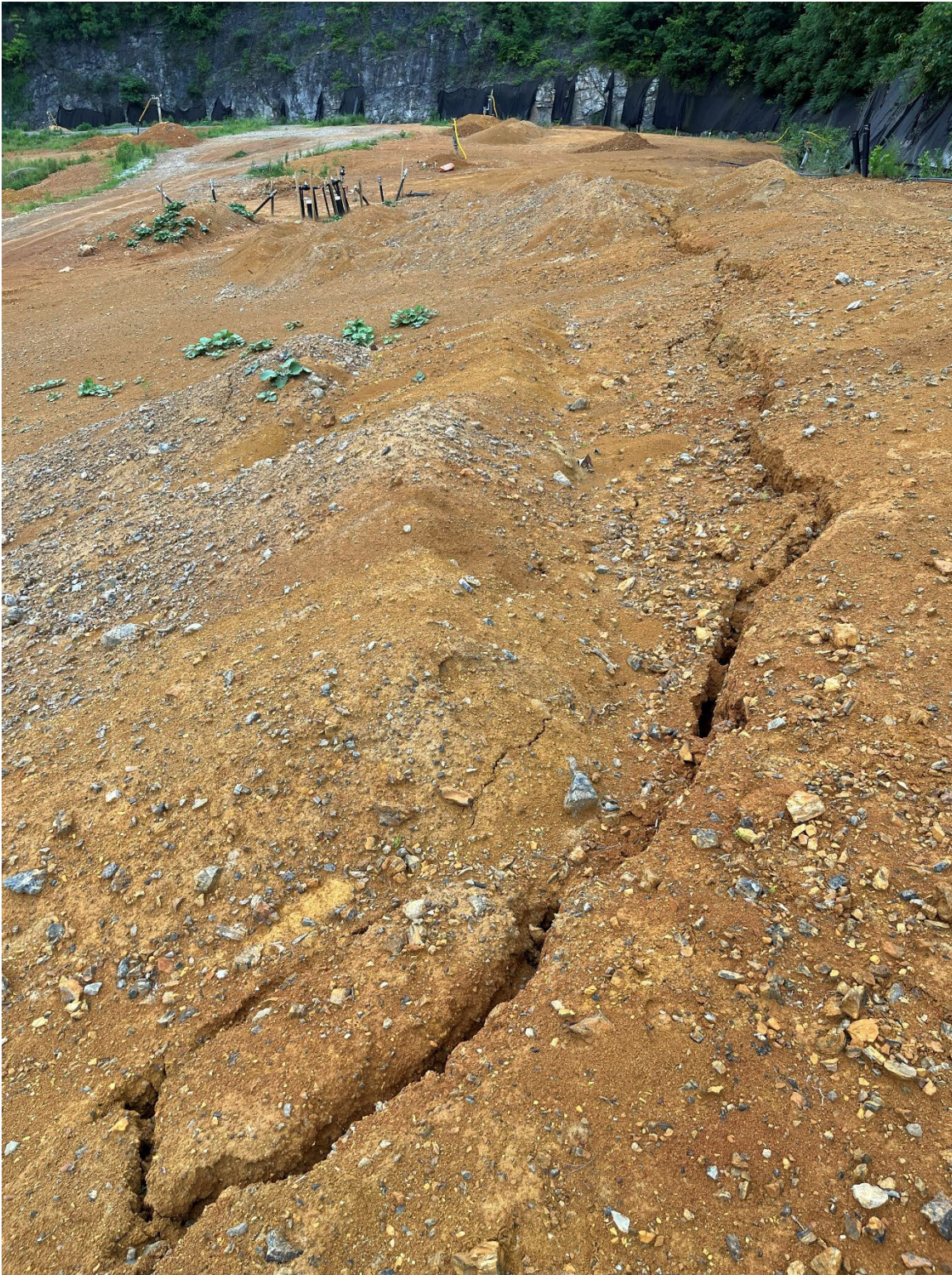
Figure 5. Settlement Crack Overview
