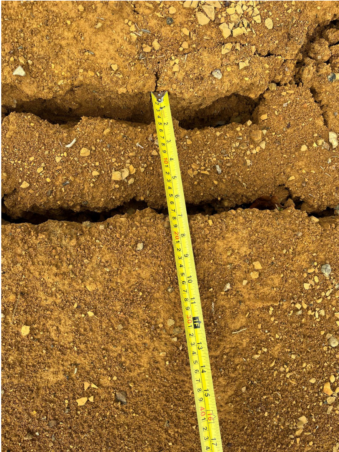
Figure 4. Settlement Crack Observed in Southwest Area Near Bench in Sidewall
