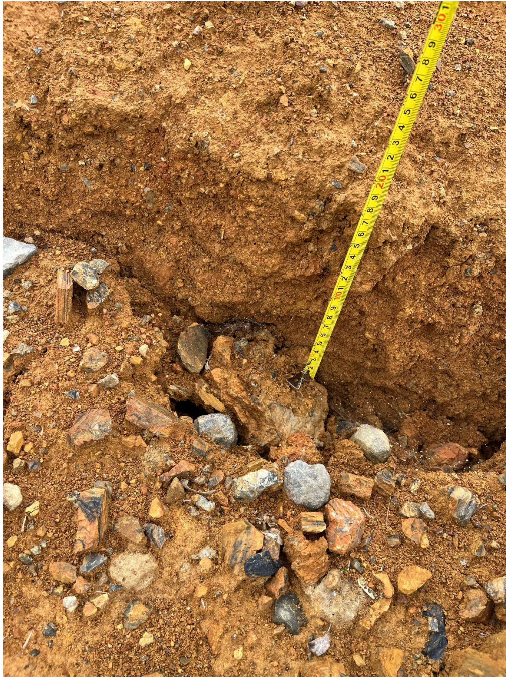
Figure 2. Settlement Scarp Observed in Southwest Area Near Sidewall Bench
