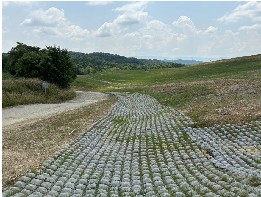
Figure 3. Vegetative growth along northern slope on 17 June 2024.
