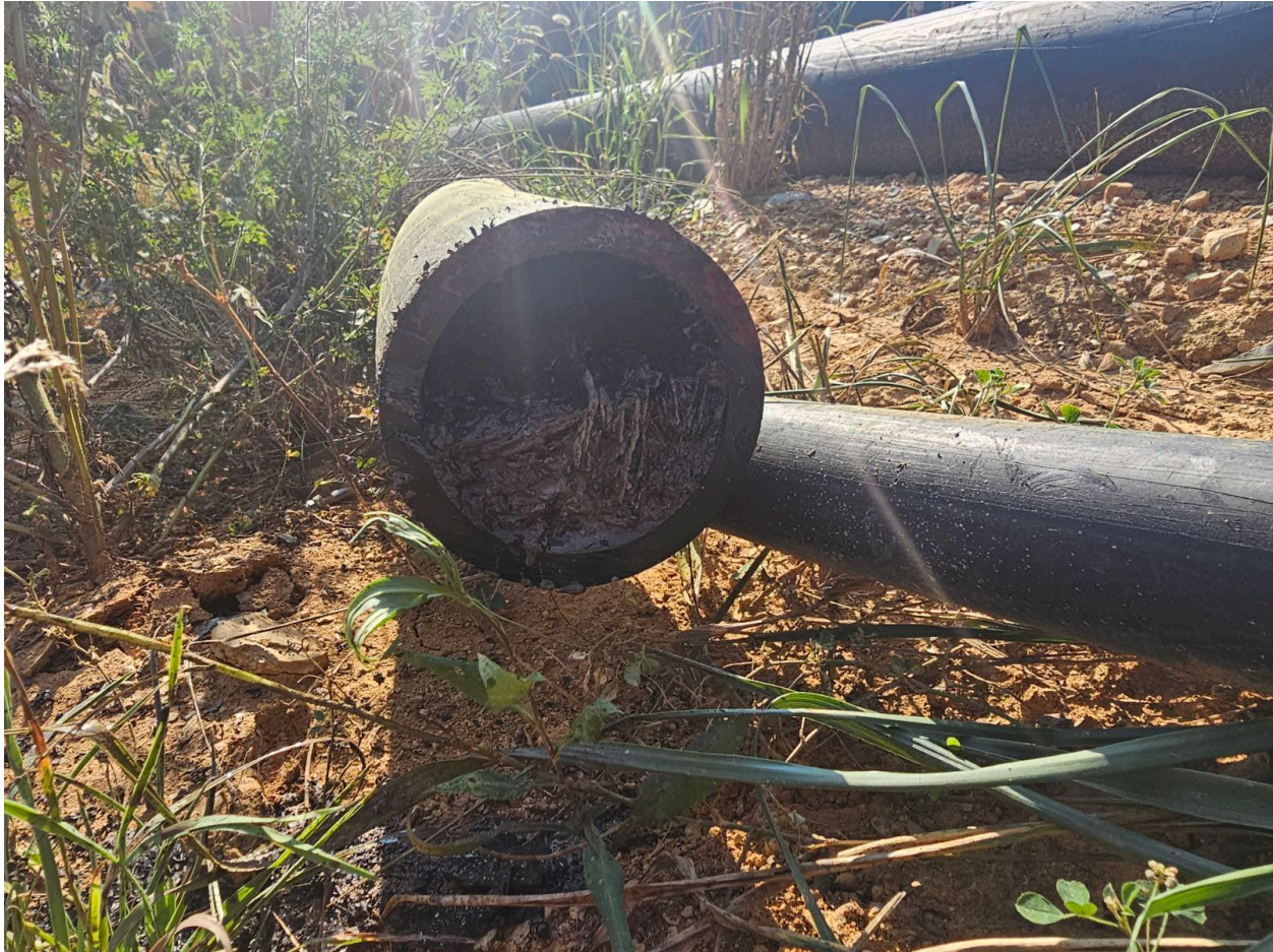
Figure 20. Solids in Landfill Gas Liquids Forcemain
