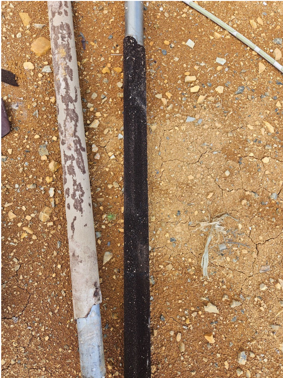
Figure 19. Solids on a Landfill Gas Liquids Extraction Pump
