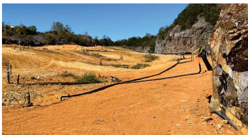
Figure 6. Phase 2 SOMS Wellhead Connections
