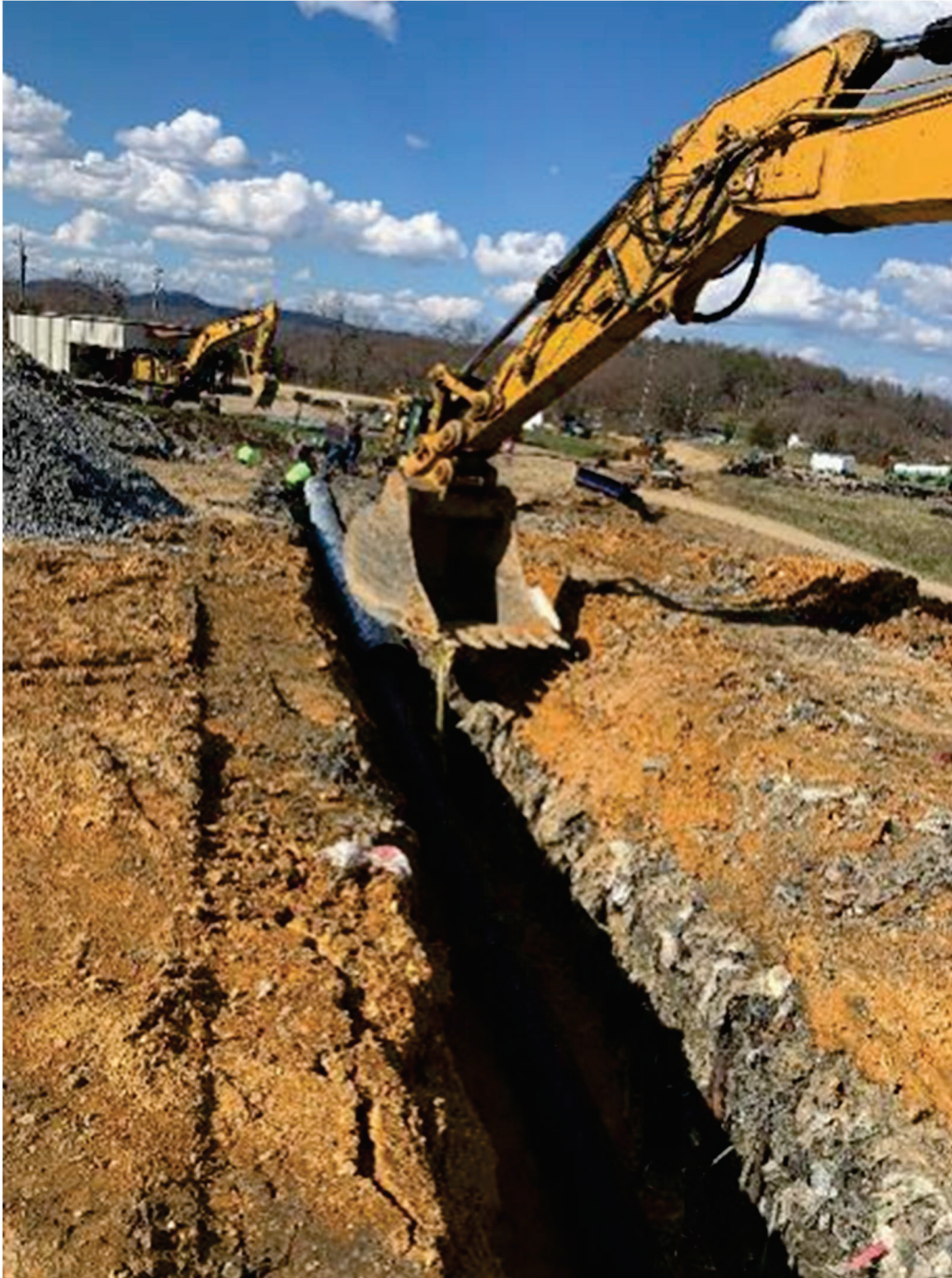
Figure 2. Landfill Gas Road Crossing - SWP No. 498 Landfill
