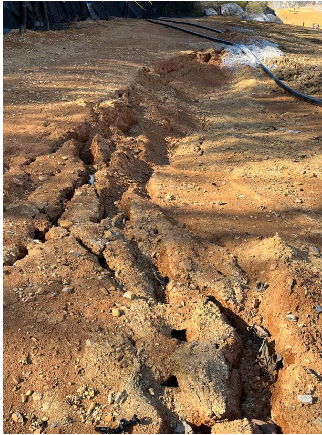
Figure 10 - Scarp and Settlement Cracks
