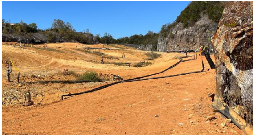
Figure 3. Phase 2 SOMS Wellhead Connections
