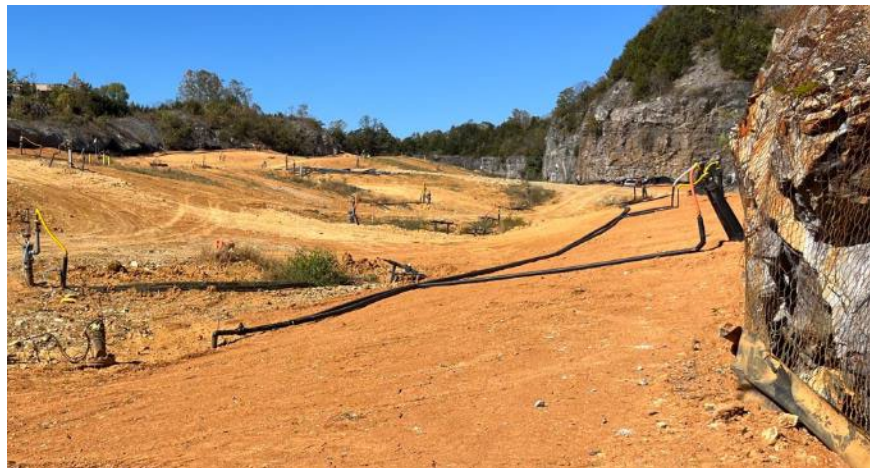
Figure 9. Phase 2 SOMS Wellhead Connections
