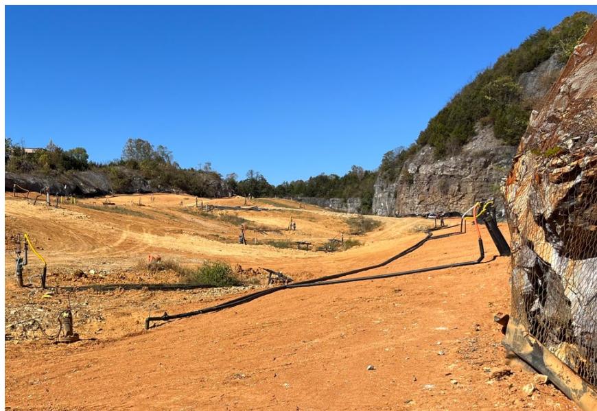
Figure 9. Phase 2 SOMS Wellhead Connections
