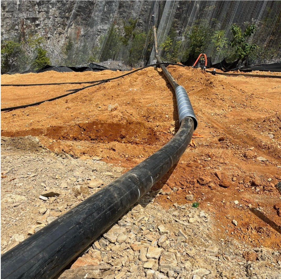
Figure 7. CMP Installation, Protecting 12" HDPE for Future Road Crossing at the SWP No. 588 Landfill
