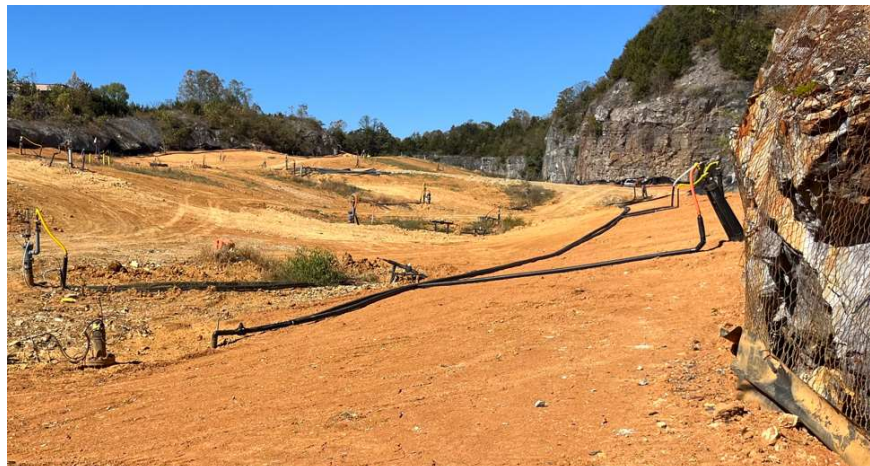
Figure 10. Phase 2 SOMS Wellhead Connections
