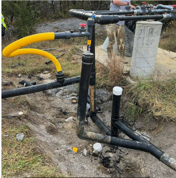
Figure 1. Manhole Wellhead Connection at the SWP No. 588 Landfill
