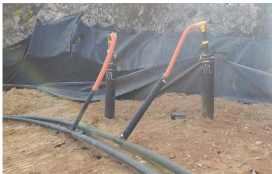
Figure 9. Phase 2 SOMS Wellhead Connections
