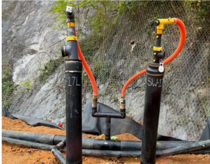
Figure 5. Phase 2 SOMS Wellhead Connections
