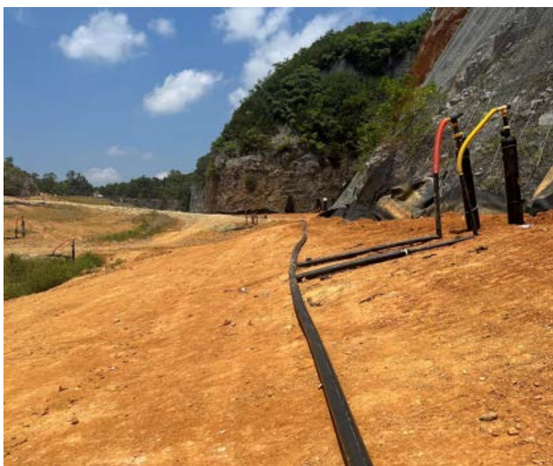
Figure 6. Phase 2 SOMS Wellhead Connections
