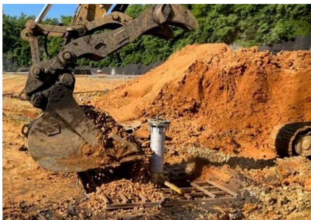
Figure 1. Stainless Steel Well Installation at the SWP No. 588 Landfill
