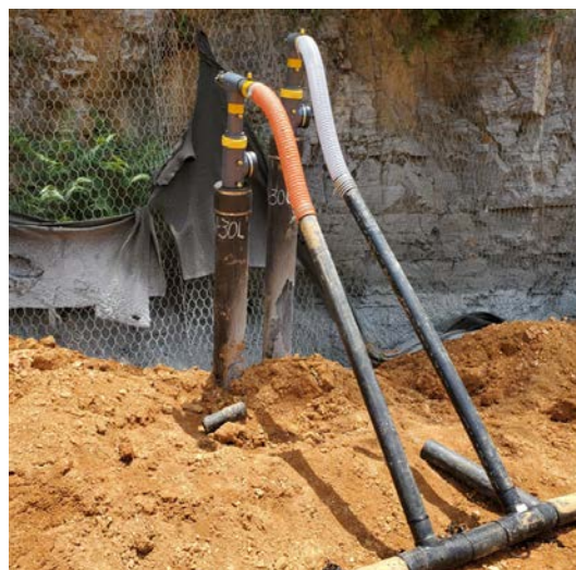
Figure 3. Phase 2 SOMS Wellhead Connections
