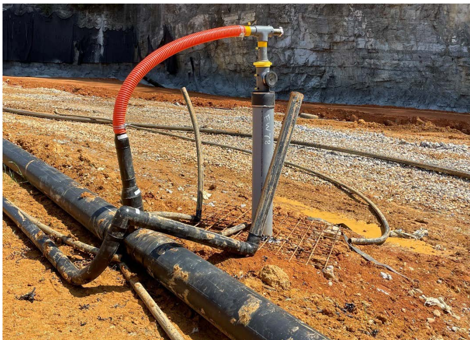
Figure 2. Perimeter Landfill Gas Extraction Well EW-78 Connected to Lateral Piping
