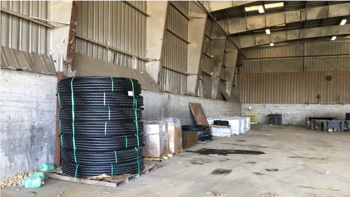
Figure 3. Landfill Gas Collection System Piping Delivered to the ISWMF
