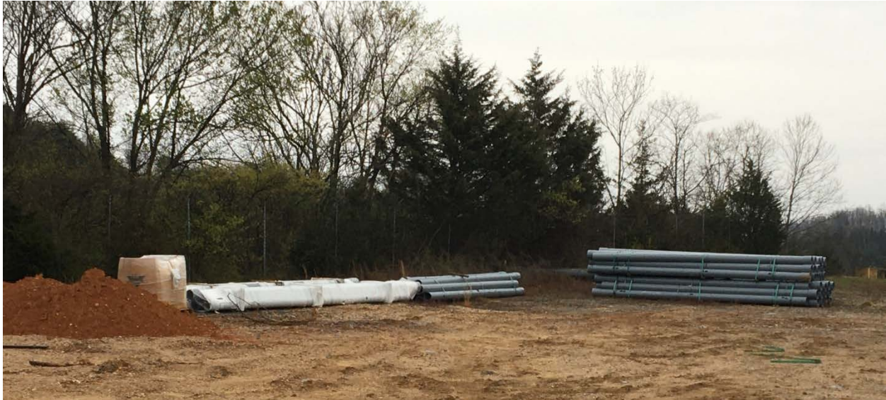
Figure 4. Chlorinated Polyvinyl Chloride Casing for Landfill Gas Extraction Wells
