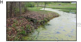
EXISTING 18"Ø RCP HALF PIPE SPILLWAY WITH UNDERLYING 12" CMP CULVERT CONNECTED TO 12"X15" STEEL BOX RISER, SEE PHOTO: RCP INV. IN: 1823.4' RCP INV. MID: 1823.6' RCP INV. OUT: 1822.8' STEEL RISER TOP: 1823.3' CMP INV. OUT: 1821.2'
