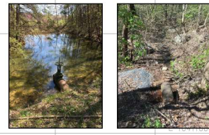
EXISTING 12"Ø STEEL PIPE OUTFALL WITH VALVE ON INLET SIDE, SEE PHOTOS: INV. IN: 1817.8' INV. OUT: 1816.8'
