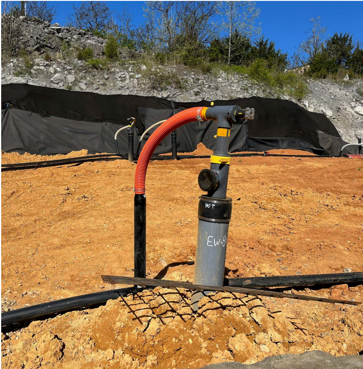
Figure 3. Landfill Gas Extraction Well EW-84 Connected to Lateral Piping
