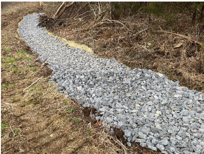
Stormwater diversion channel and trench berm with sediment removed, erosion control matting in place, and aggregate placed & spread.
