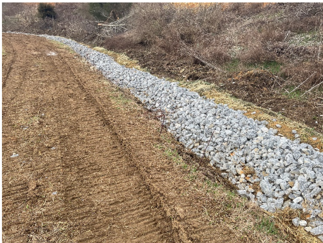
Stormwater diversion channel and trench berm with sediment removed, erosion control matting in place, and aggregate placed.
