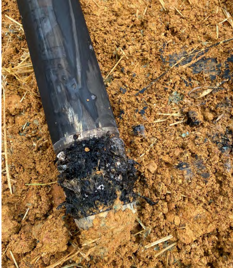
Figure 11. Material Clogging Landfill Gas Well Dewatering Pump
