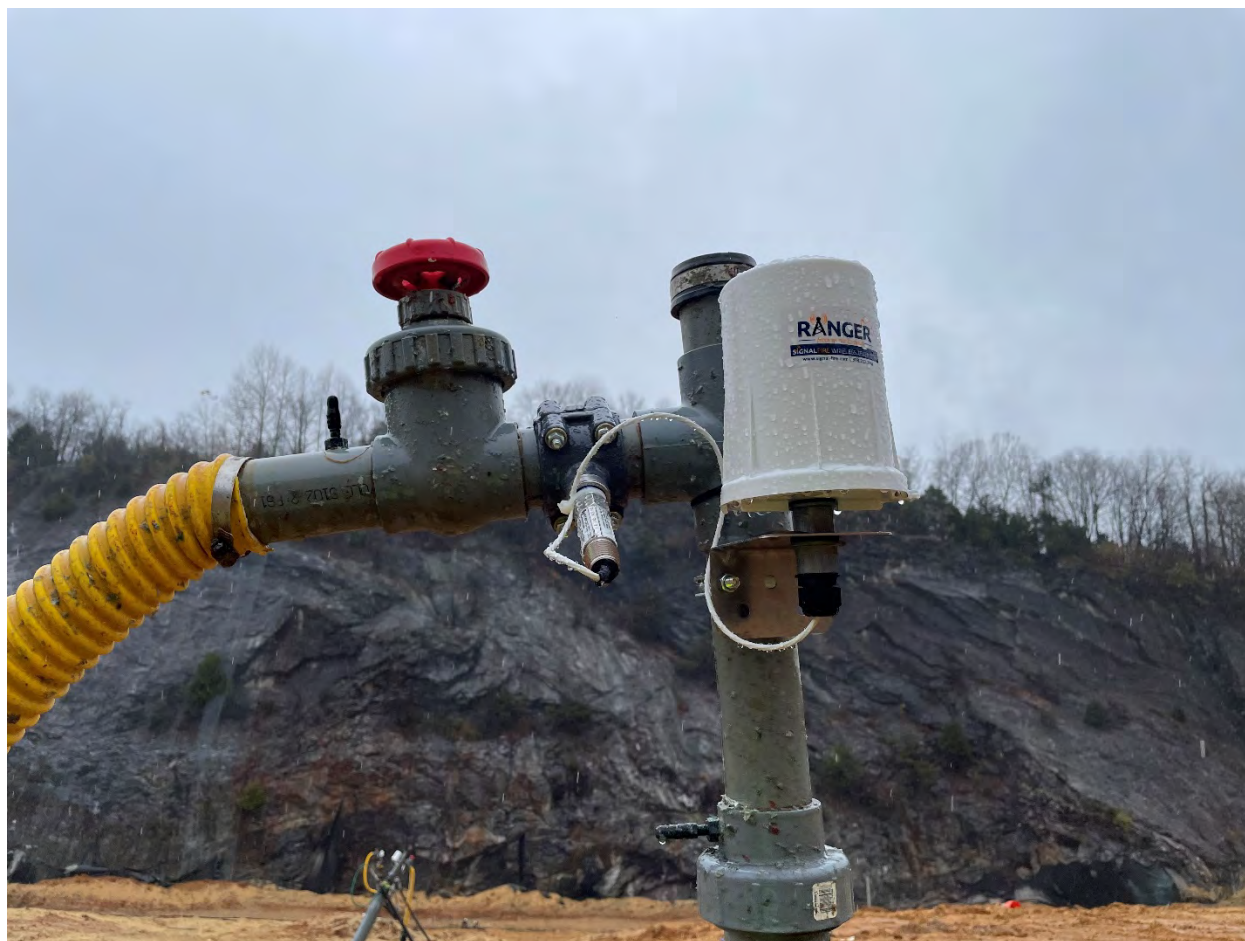
Figure 4. Wellhead Temperature Sensor after Installation
