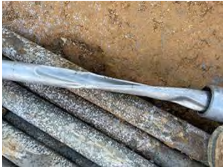
Figure 10. TP-1 Casing Damage
